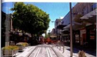
Tracks were laid in the Cashel Street Mall during its refurbishment in 2005.
