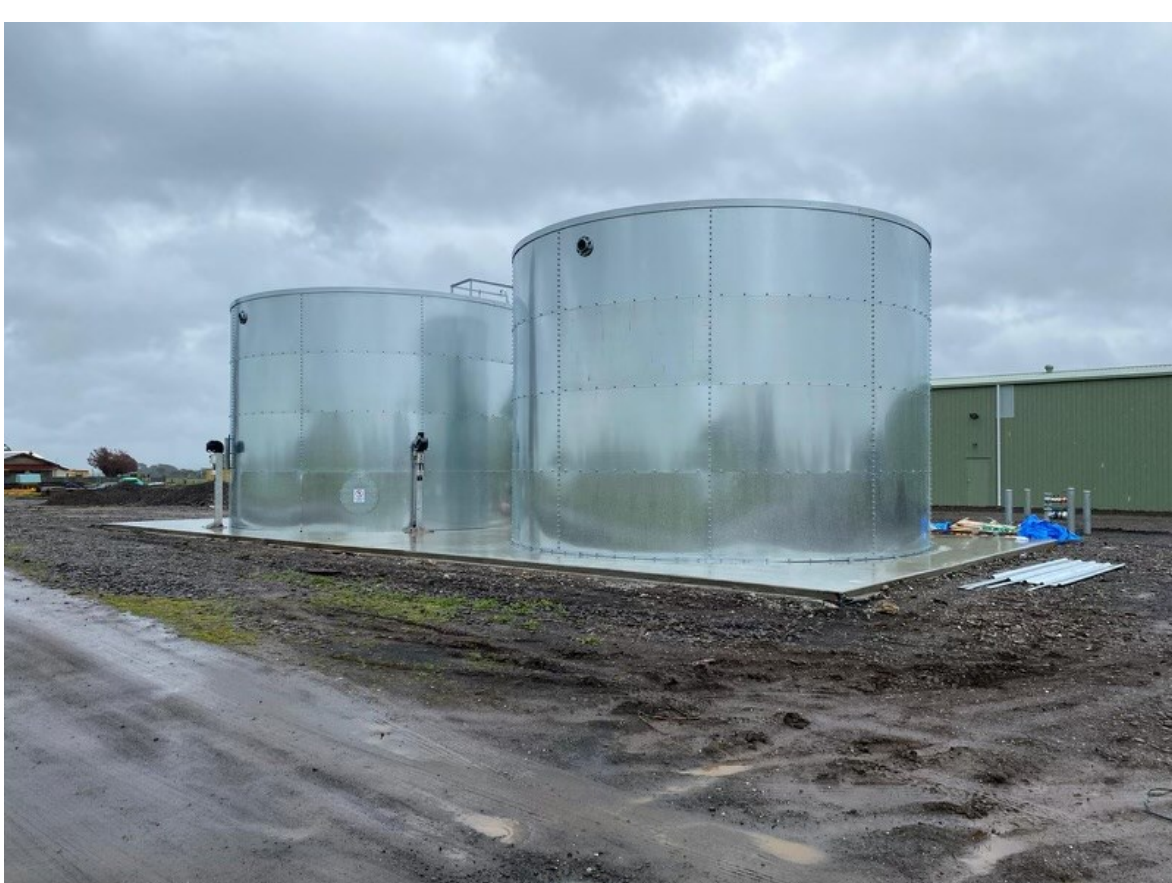
Fire Protection water storage tanks.
