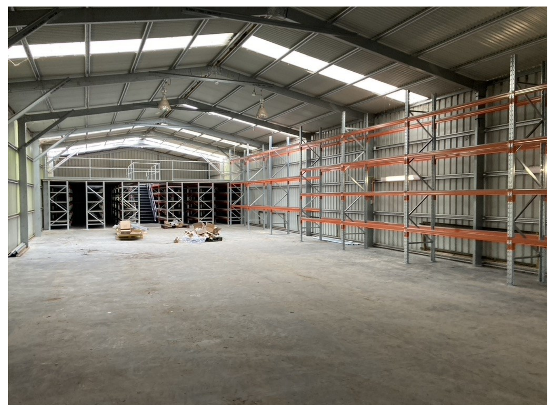
Installing pallet and storage racking in the 2010 built shed that had been used for tram storage. This will also be used for COTMA parts storage.
