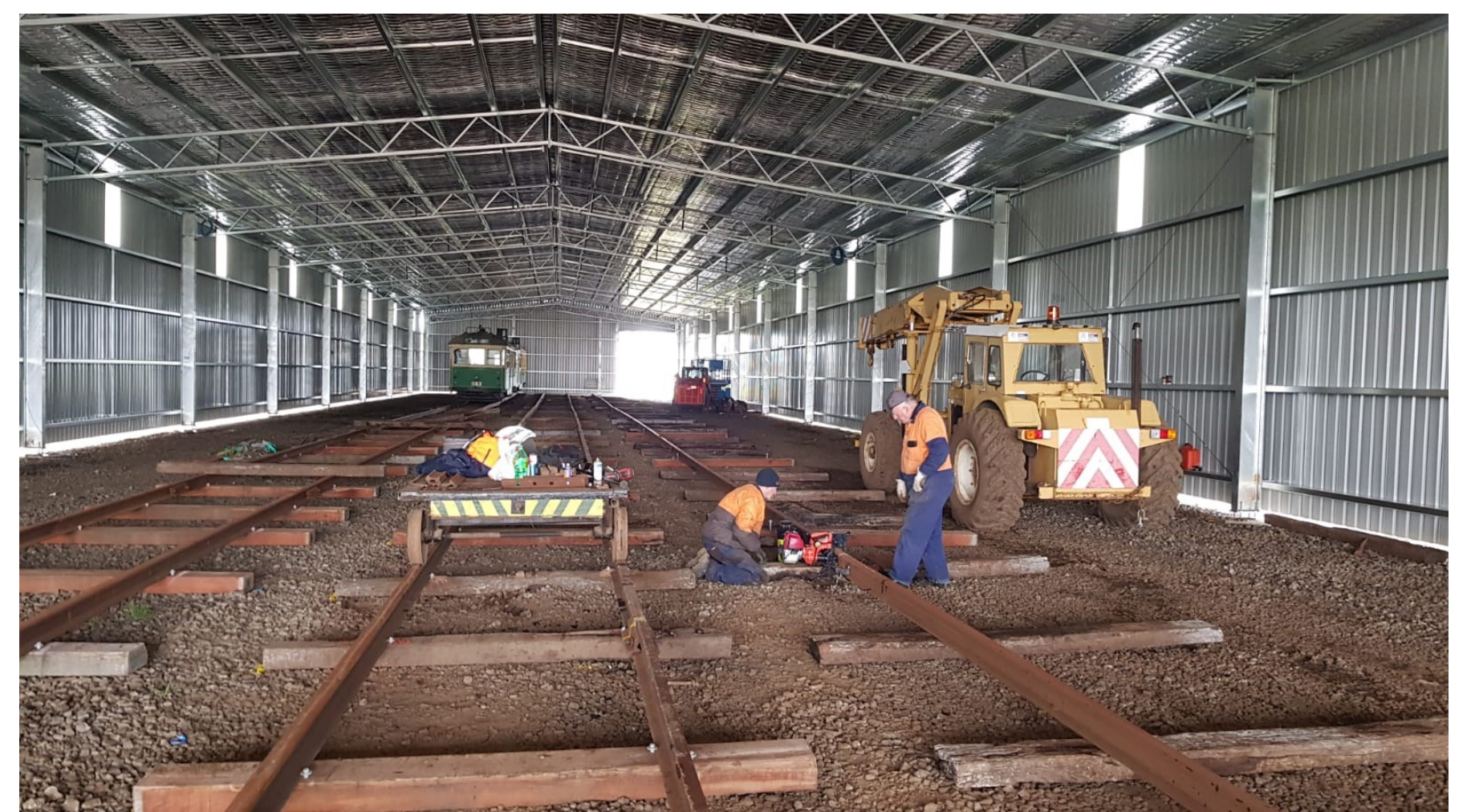
There are five separate tracks with a tram right at the back.
