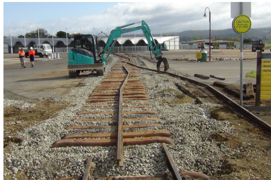
Photo: Graeme Davis Rails removed from the timber sleepers and set aside were moved back to the line of the track.
