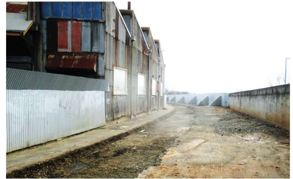
Photo: Graeme Davis Old track bed removed ready for laying a new track bed and ballast.
