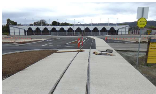
Photo: Tony Weston Completed trackwork with sleepers covered in concrete and asphalt, with the railway turntable and a tribute to the former locomotive roundhouse behind.
