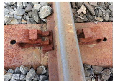
Photo: Tony Weston Detail of the clips holding the rails to steel sleepers.
