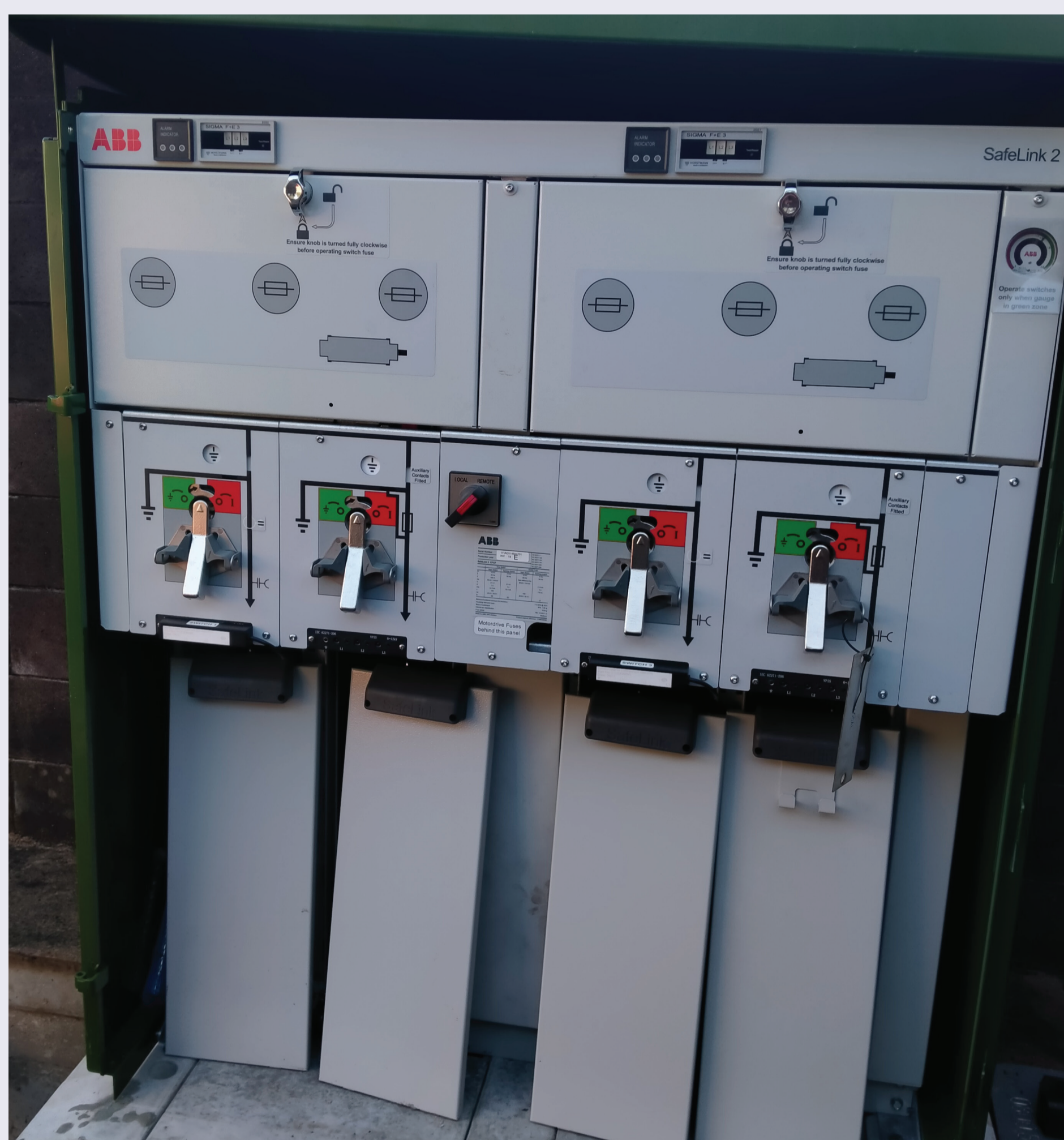
From 1980 onwards with the closure of the Auckland trolley bus system, MOTAT had its own traction power supply installed, using a mercury arc rectifier, the power now coming direct from the supplier, Vector. Outside the MOTAT Main Entrance are these 11kv A.C. fused switches controlled by Vector.
