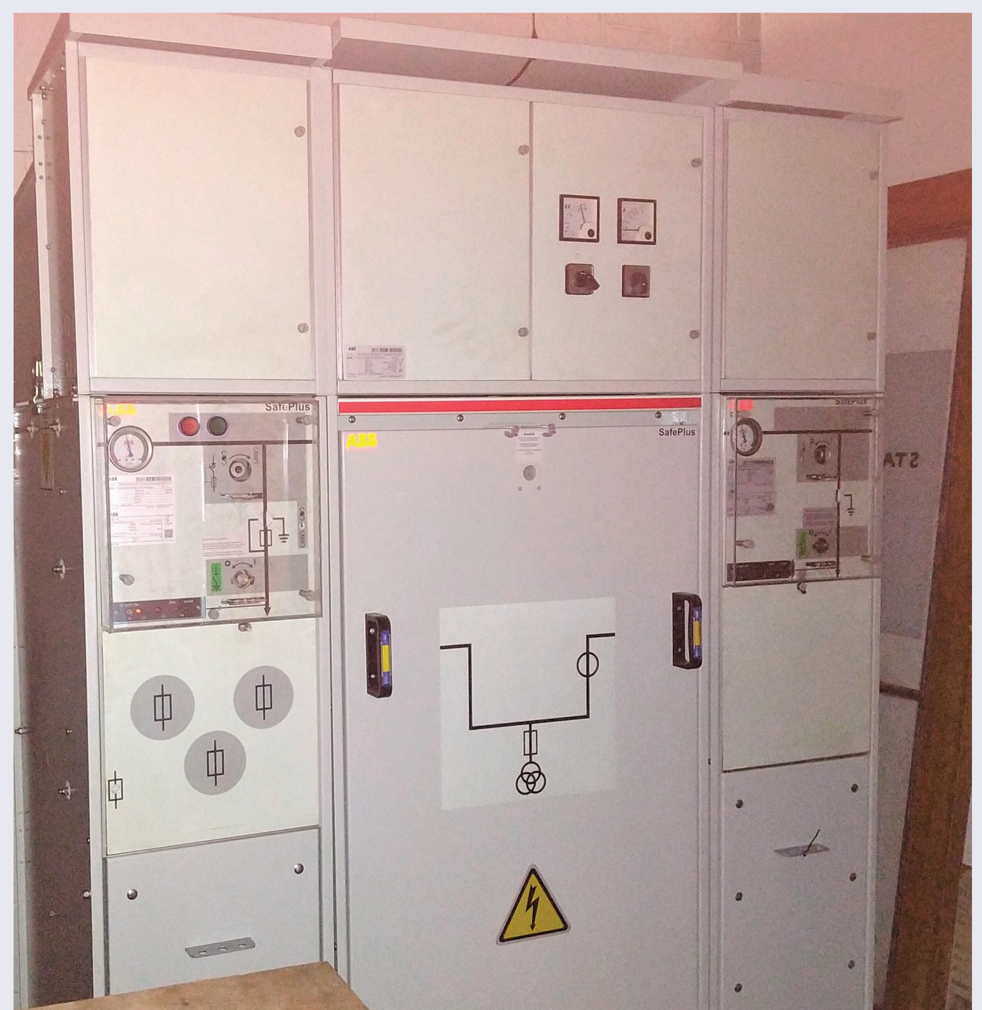
When the museum's new traction supply was set up in 1980, it was protected by a large oil-filled circuit breaker. To maintain absolute protection, this oil-filled circuit breaker was replaced in early 2023 by modern solid-state fused switch unit, which included a reliable metering system for power consumption charges.
