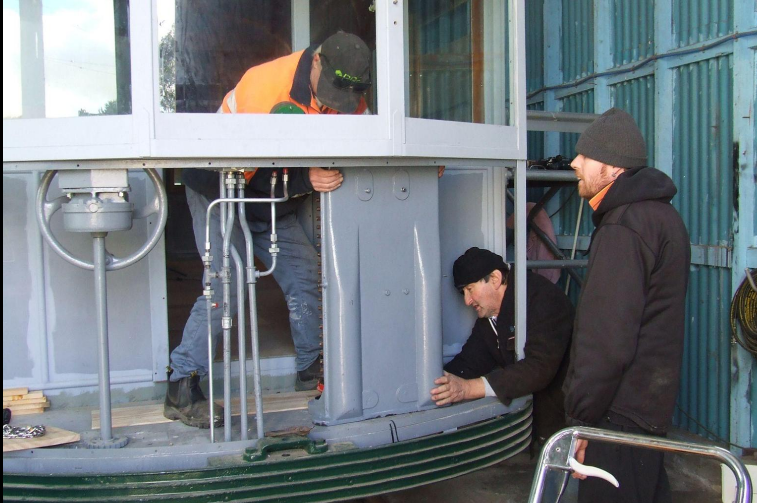
Fitting overhauled M&MTB Q2CK1 controller
